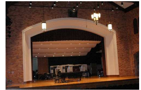
Fire sprinklers in Akin Auditorium
