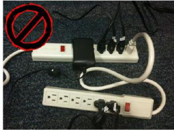
Improper "daisy chained" power strips; power strips must be plugged directly into an outlet.
