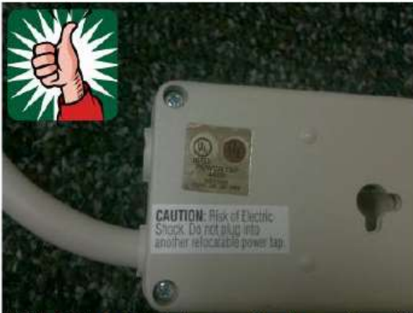
UL Listed sticker on the back of a power strip; all power strips, multi-outlet adapters, extension cords and UPSs must be UL Listed.
