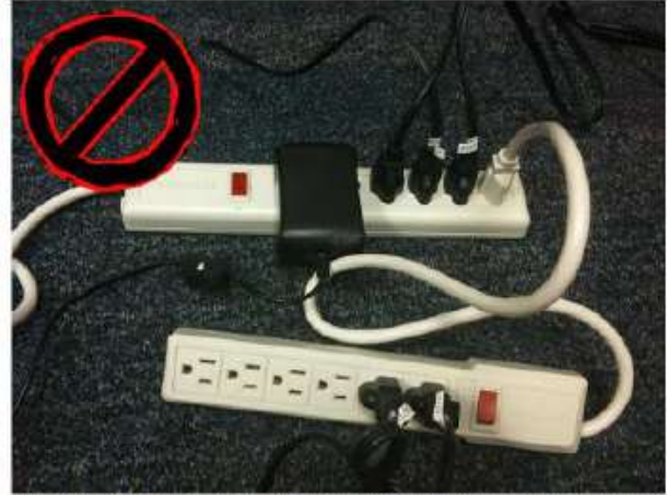
Improper "daisy chained" power strips; power strips must be plugged directly into an outlet.
