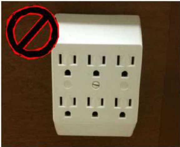
Prohibited multi-outlet adapter; multi-outlet adapters must have resettable circuit breakers.
